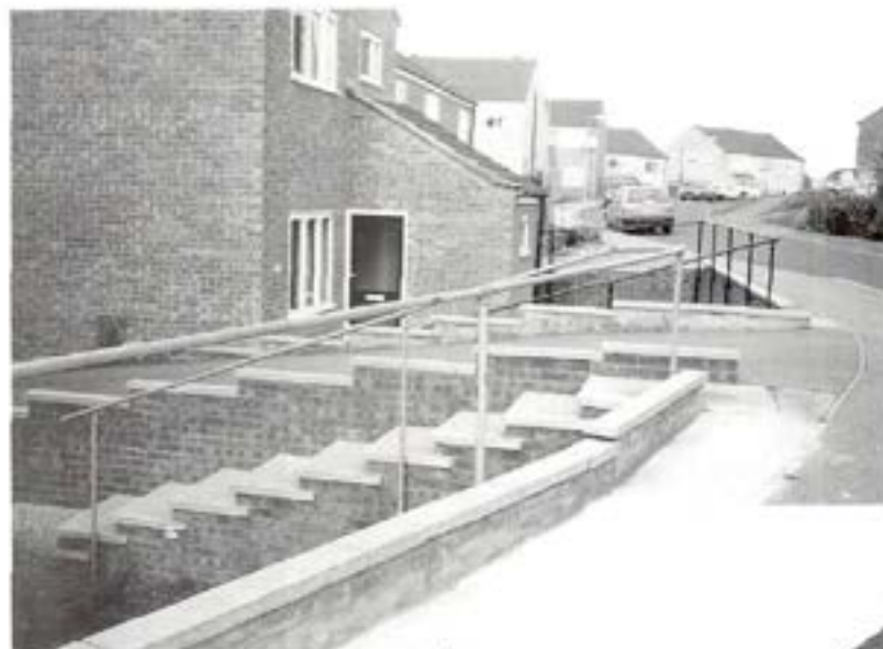
▲ Lack of attention to detail
